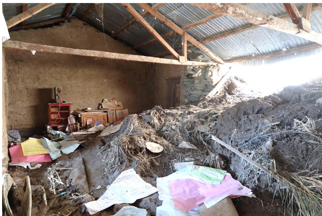
School at Borta after landslide
