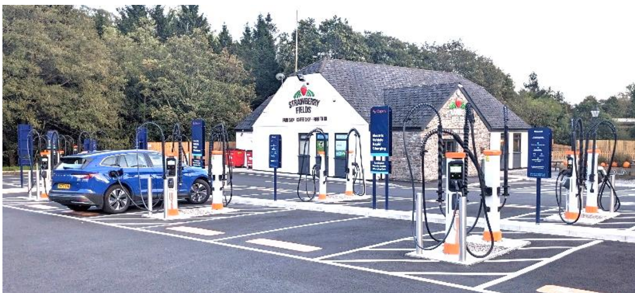
The charging point at Buckfastleigh
